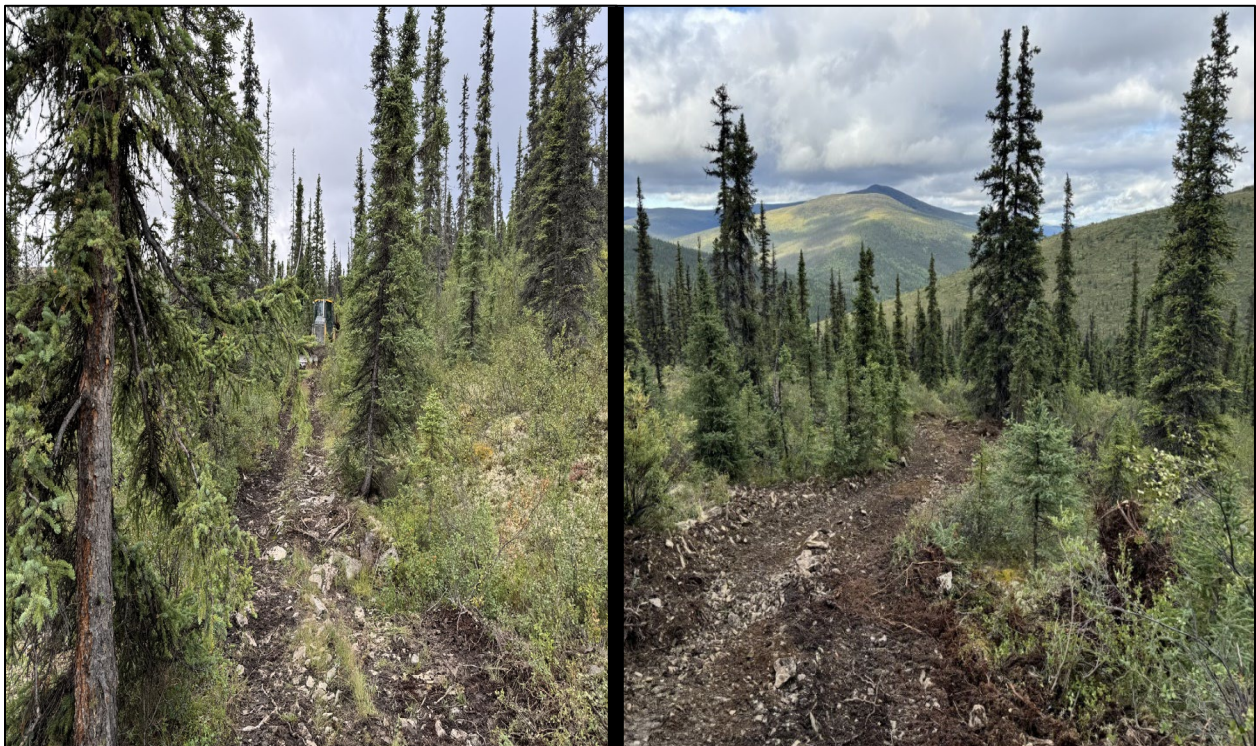
Figure 2. Before and after photos of trail work to reduce erosion and improve access in upper Harrison Creek.
