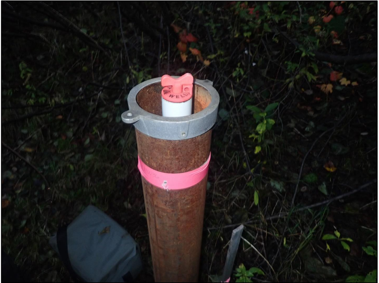
Photograph 2-9. MW36 frost jacked with collapsed PVC, 9/6/2024
