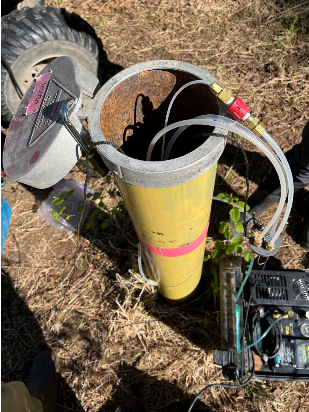
Photograph 2-2. MW54 tubing sticking out from the well after pump got stuck during transducer install, 6/4/2024.
