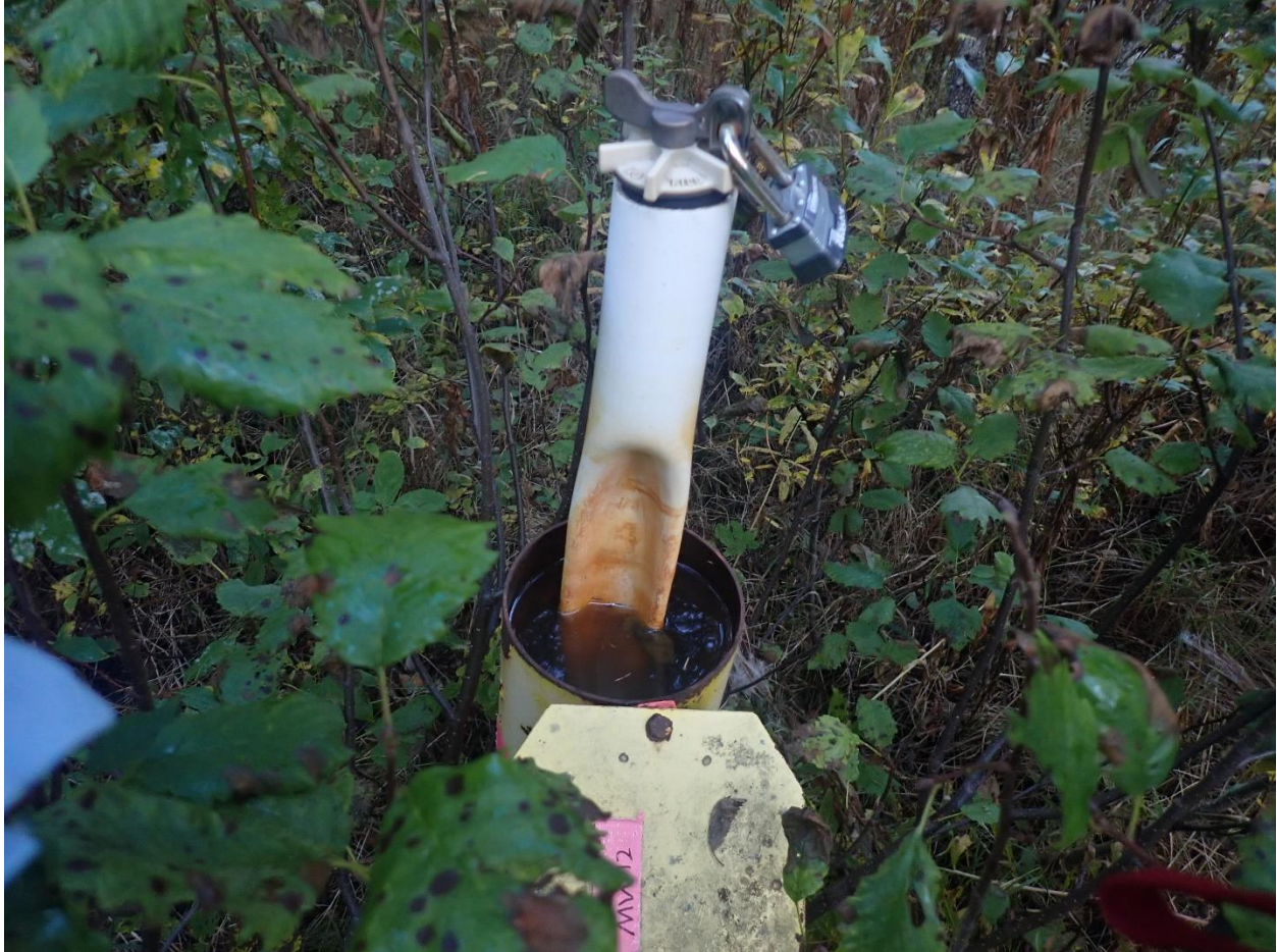
Photograph 2-10. MW12 frost jacked with collapsed PVC, 9/6/2024.
