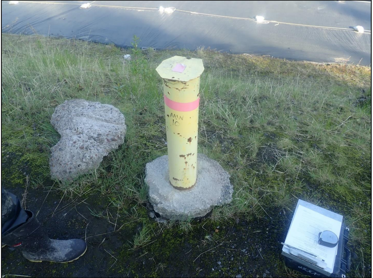
Photograph 2-8. Settling of soil and separation of the ground surface around the concrete base of MW10, 9/09/2024.
