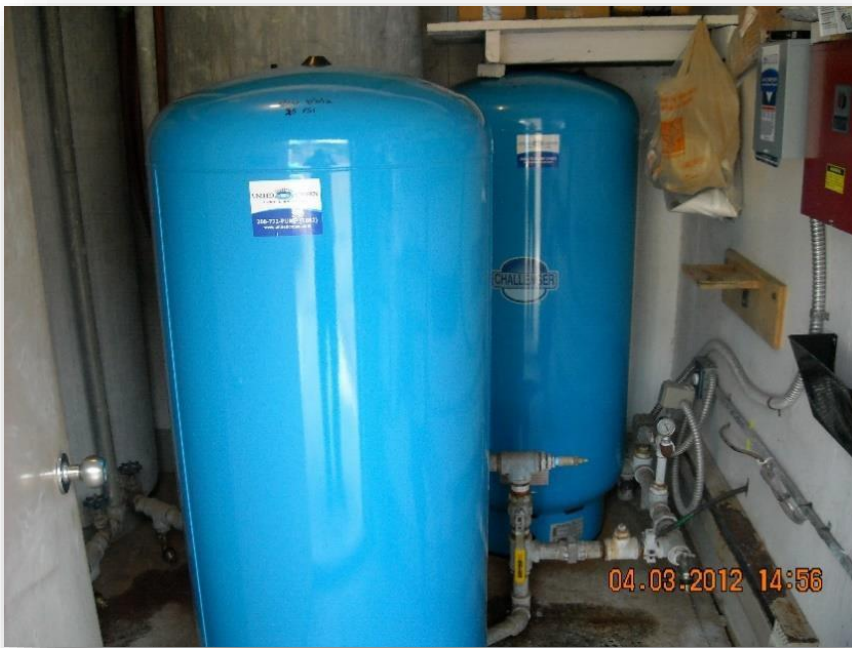
Figure 5: Current pump house with retrofitted high-pressure tanks in 2012.
