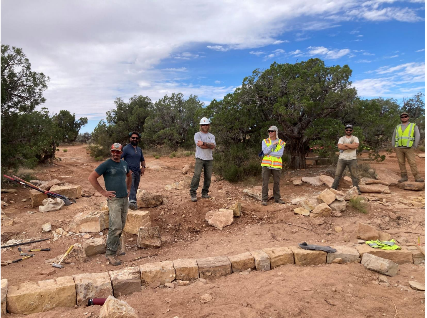
Saguaro NP Trail Crew Constructing a new accessible trail from the parking lot to the first overlook at Painted Hand Pueblo.
