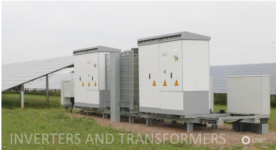
Figure 7 Photographs of a Typical Power Conversion Station/Inverter
