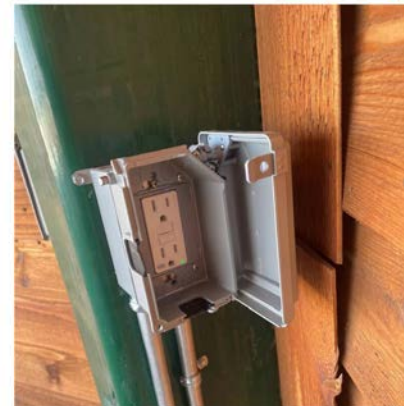
GFI Electrical Outlet at Rob Jagers Campground
