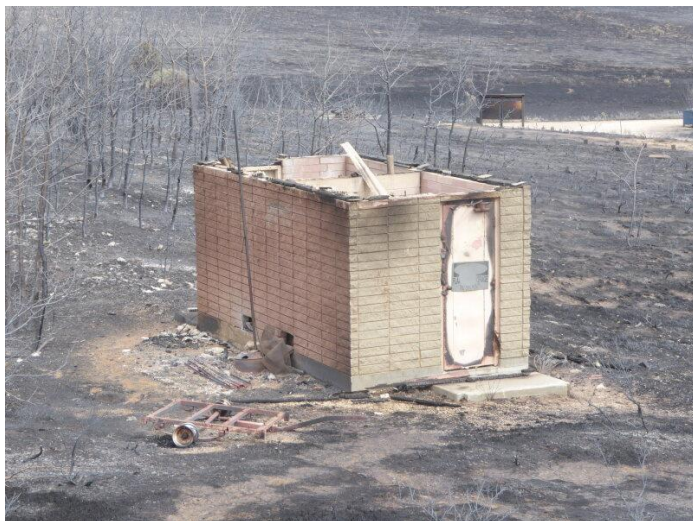
Wildhorse burned vault toilet
