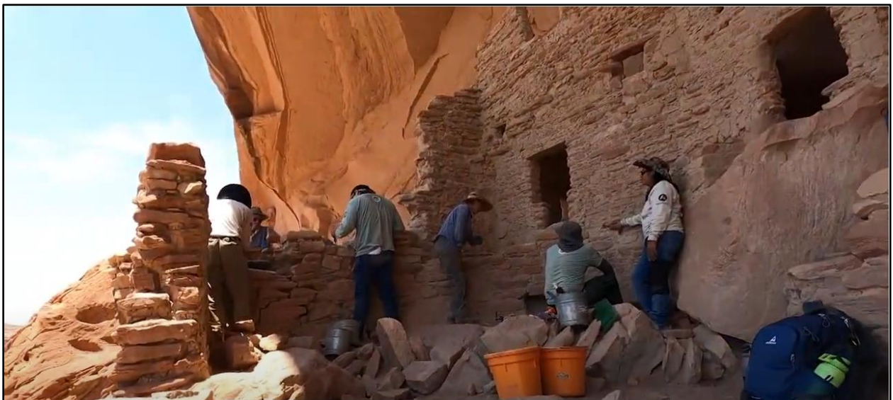
Figure 4: An Ancestral Lands Corps crew works to stabilize the River House in Bears Ears NM.
