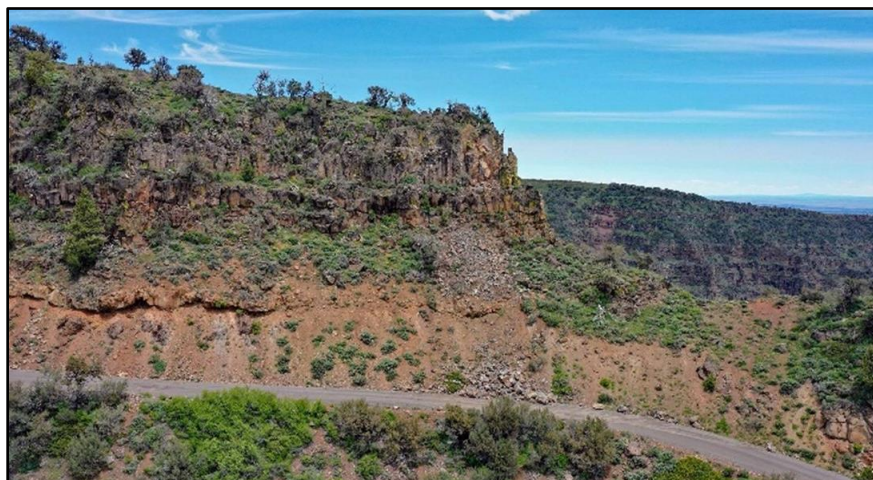
Rockfall on the Rooster Comb section of the South Steens Loop Road
