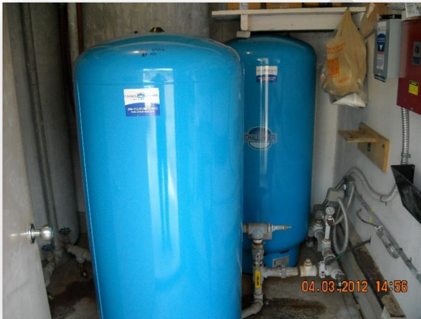
Figure 5: Current pump house with retrofitted high-pressure tanks in 2012.
