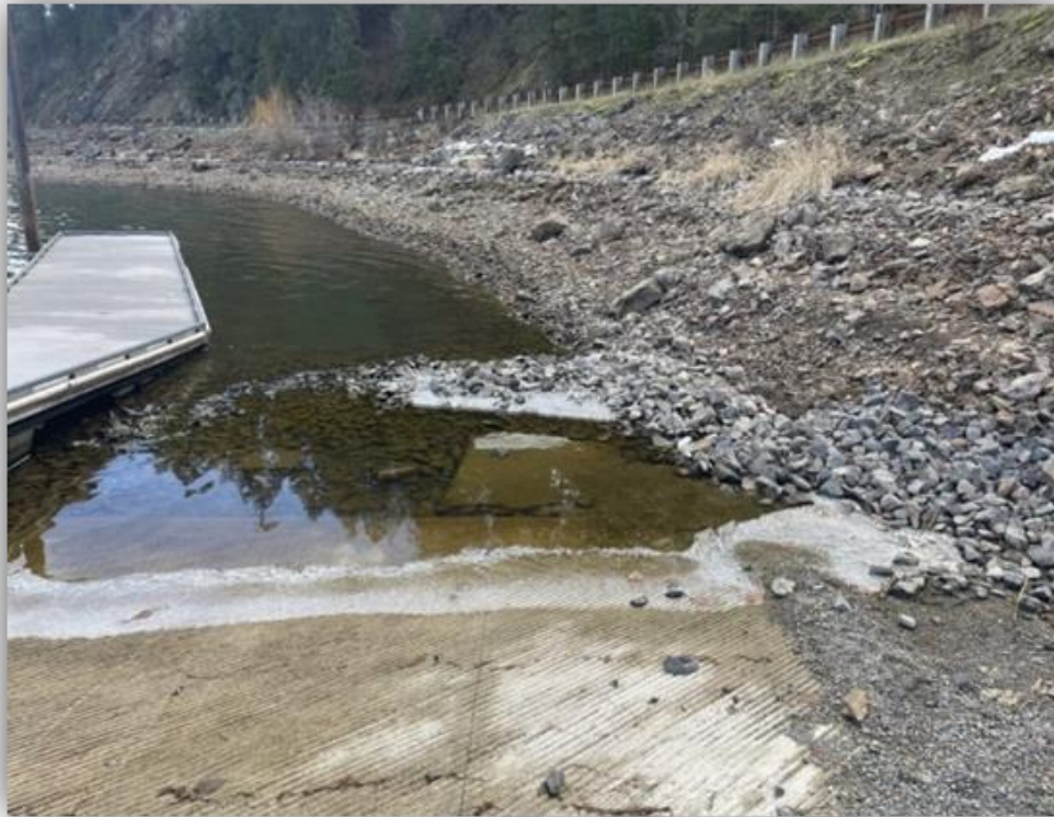
Figure 7: Riprap creating a launch hazard at Mineral Ridge Boat Ramp
