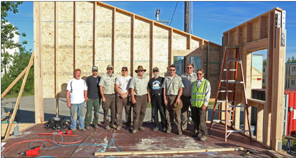
(left to right) BLM AFS carpenters Al Schultz and Bronson Singh; FWS employees Shane Miller, Kody Goodge, and Jim Donaldson; BLM AFS carpenter Jeffrey Perkins; FWS employees Kyle Goodge; Joe Whatley, and Steven Howerton.
