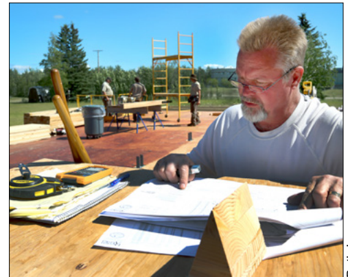
(top) BLM AFS carpenter Jeffrey Perkins holds things in place while FWS employee Joe Whaley of Cypress Creek National Wildlife Refuge in Illinois nails beams together. (above) BLM AFS carpenter Al Schultz checks the construction plans in Galena.
