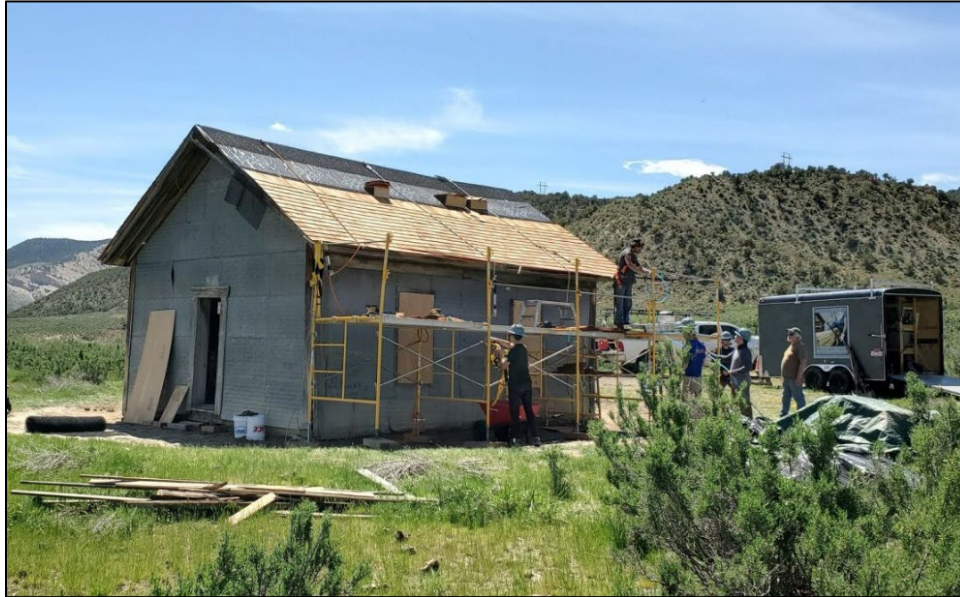
Figure 14. HistoriCorps' fieldwork underway for Phase I initial stabilization of the Yellow Creek Schoolhouse, May 17, 2023.
