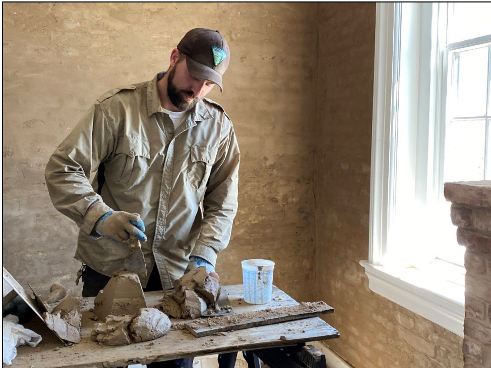
BLM staff member working on the restoration of the historic work room
