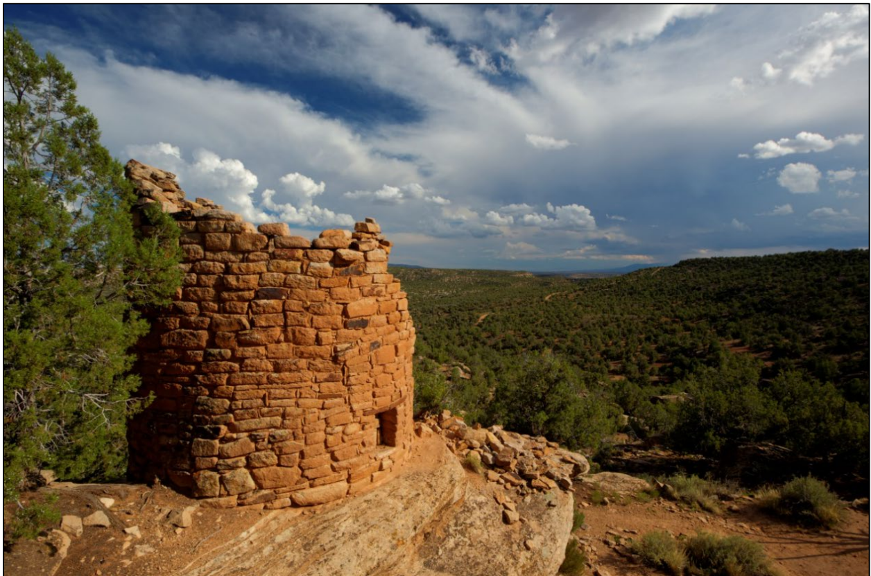
Tower A at Painted Hand Pueblo, one focus of this year's stabilization work under the interagency assistance agreement between CANM and preservationists at Mesa Verde National Park.
